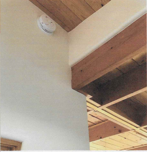
SMOKE/CO2 DETECTOR HALLWAY/LIVING ROOM/KITCHEN
